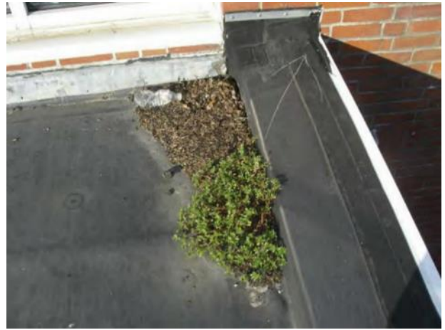
Accumulation of debris – clogged-gutters
