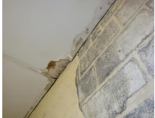
Interior leakage/damage inside roof area
