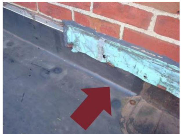
Missing/deteriorated copper flashing at the rising wall
