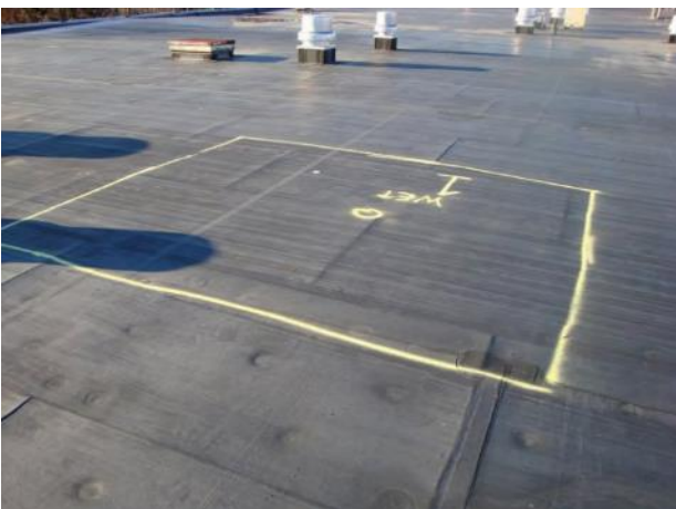
Wet-insulation over classroom. A hole/puncture in the membrane is the source of the damage.
