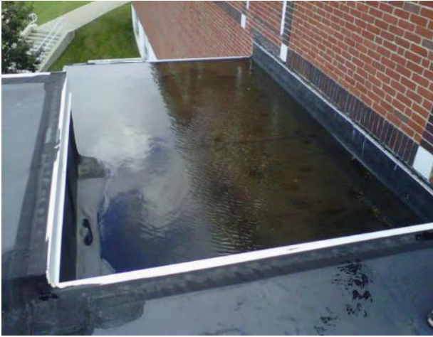
Standing-water (ponding) on the roof area
