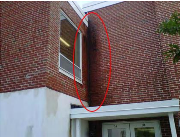
Leakage from/behind/under roof/damaging/staining the brick
