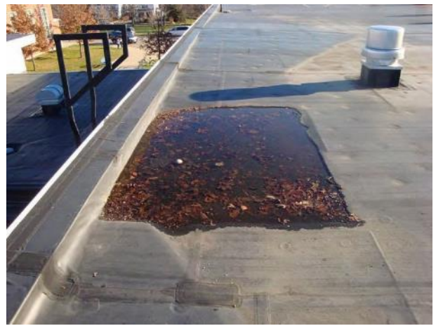
Standing-water (ponding) due to a covered-over roof drain
