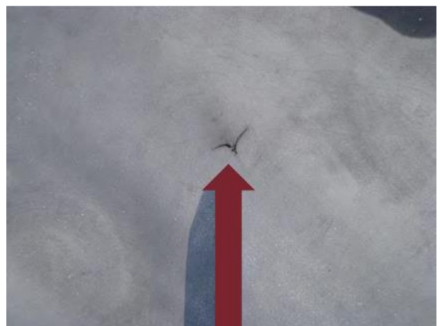
Close-up of the small hole responsible for the wet-insulation.
