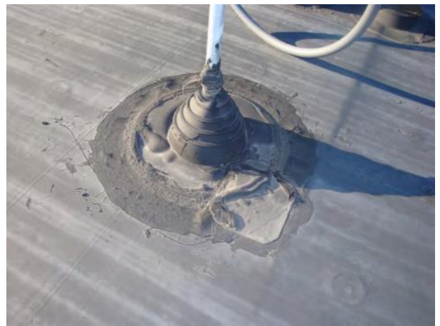
Poorly-installed flashing-boot detail at an electrical feed
