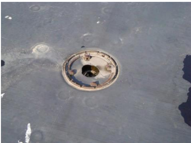
Missing roof drain strainers
