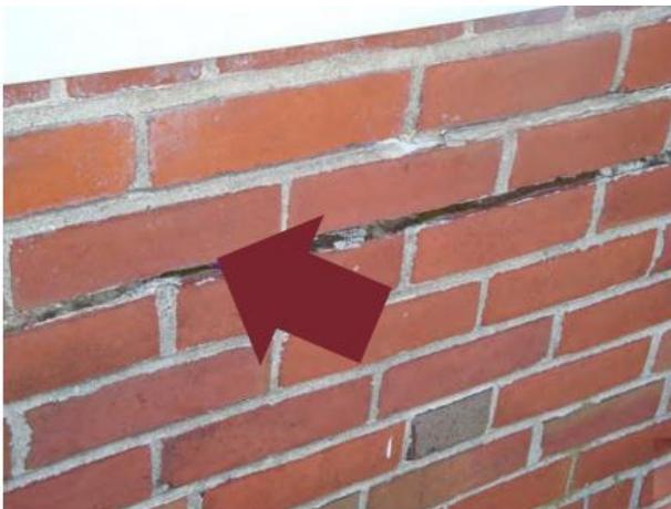
Missing/deteriorated mortar joints
